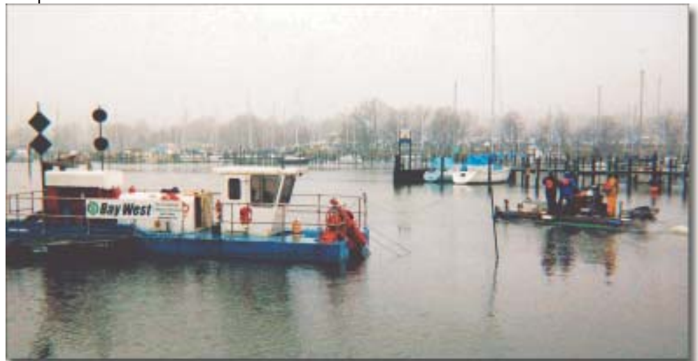
Bay West used an Ellicott 370 hydraulic cutterhead dredge to perform maintenance dredging of this navigation channel for the Baltimore District.
