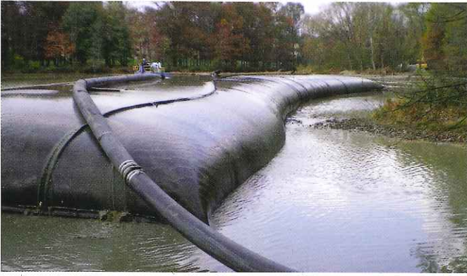
Geotextile tubes being used to dewater dredged material and establish a habitat for wetland vegetation.
